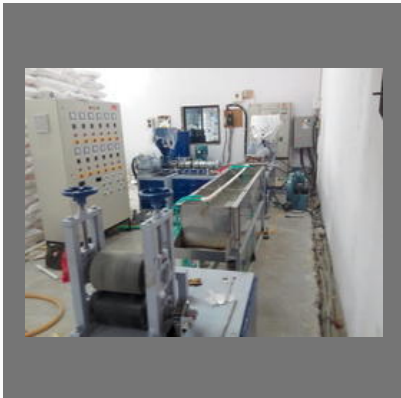
SOFT PVC Garden Pipe Plant
